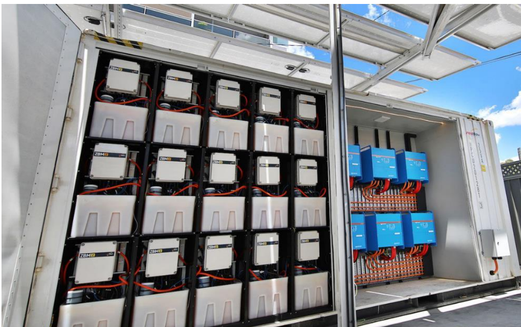
Figure 11 Typical flow battery installation showing three rows of stacked cells. Photo credit: Redflow Limited
